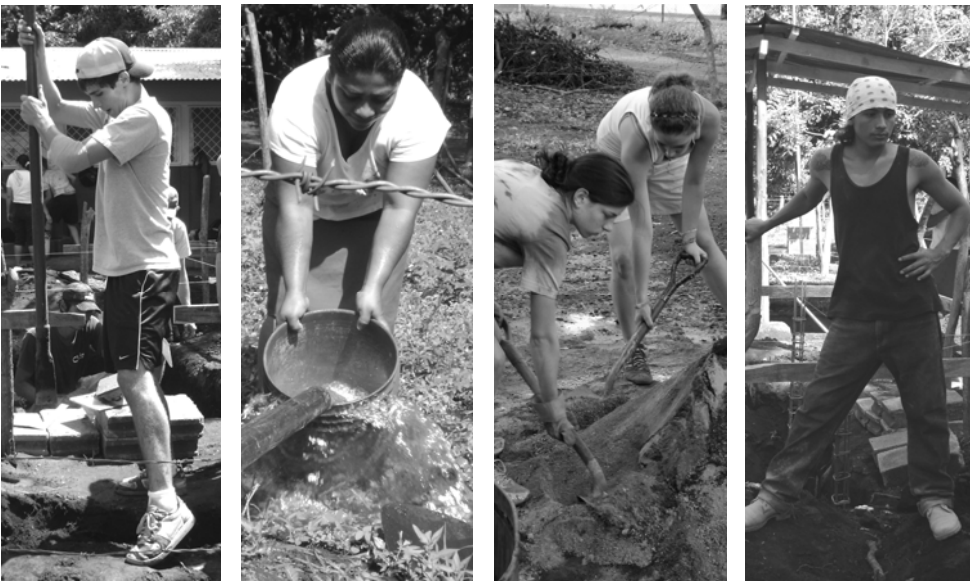
Images from the June 2008 construction of a water system for a school and health clinic in Goyena. The project was made possible by funds from South Congregation Church in Middletown, CT; the labor of Hopkins High School students from New Haven; the know-how of engineers from León; and the organization and coordination efforts of community members.
